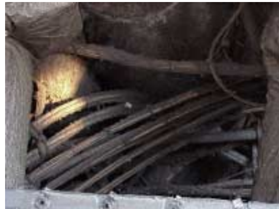
Figure 2-6: L1011 Under Floor Panels showing excessive dust and lint build-up.
