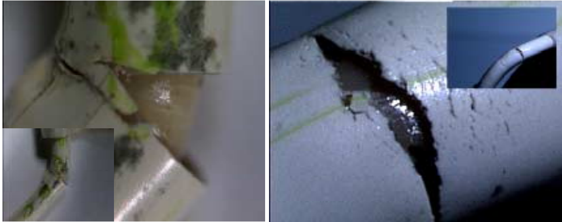
Figure 4-10: 747 wire from section ECH-2 Zone 10 (alkene-imide polymer) showing cracked insulation from mandrel bend (left); non-aircraft wire (alkene-imide polymer) that also cracked (right).
