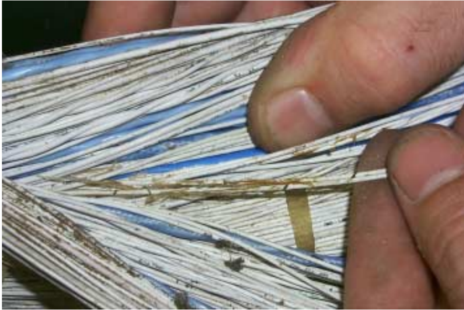
Figure 4-1: A300 LCL Midspan (FEP, polyimide insulation) bundle with breached wire as found from DelTest™.
