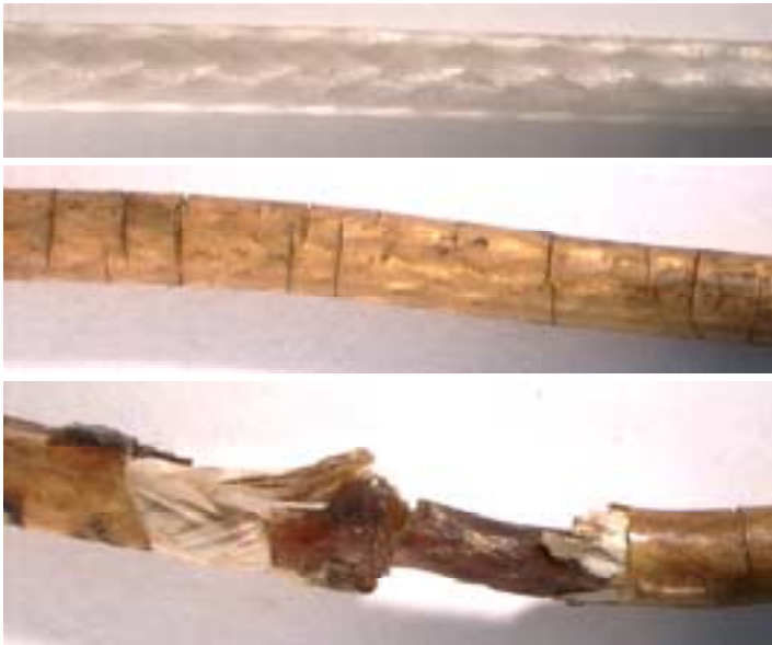
Figure 4-17: Multiple pictures (all at 3.5X) of the same DC-9 (2) wire from section ENL (Nylon/Glass/PVC) illustrating the range of conditions observed.
