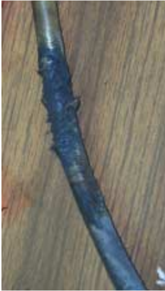
Figure 4-15: Burnt DC-9 (EPF) wire found by the DelTest™, that was inside a steel conduit and visually impossible to detect.
