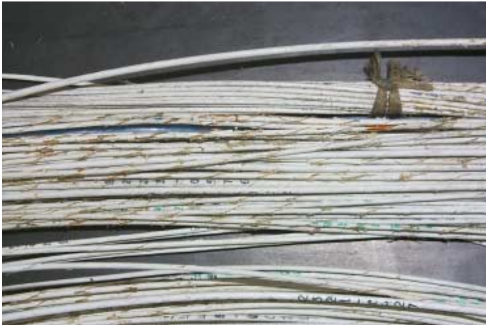
Figure 4-2: Picture of A300 LCL Midspan (FEP, polyimide) bundle in region where the topcoat is cracked and has unknown flakes on numerous wires.
