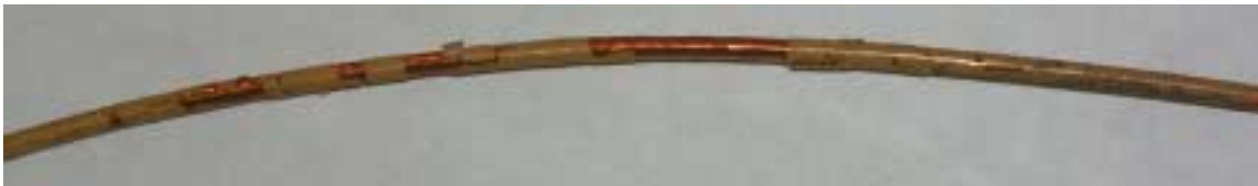
Figure 4-22: An L1011 wire from section RW LE (polyimide). The topcoat (yellow layer) is flaking off, cracked, and missing in places, exposing the taped insulation.
