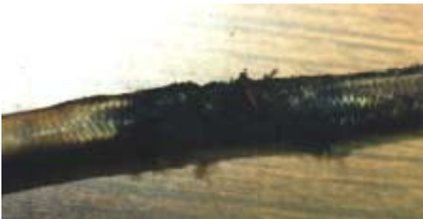
DC-9 Tail Cone Power Feeder removed from conduit
