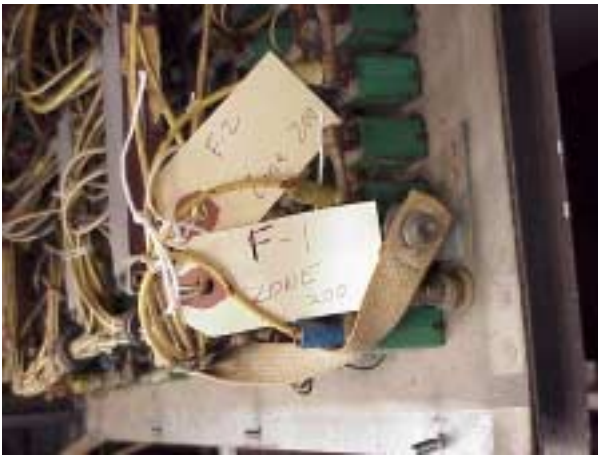
L1011 Circuit Breaker Panel
