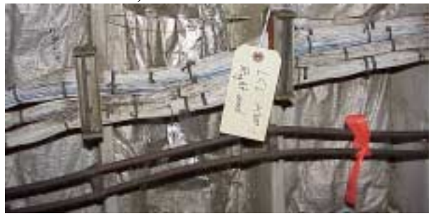
A300 EE Bay, LCL specimen where delamination was discovered
